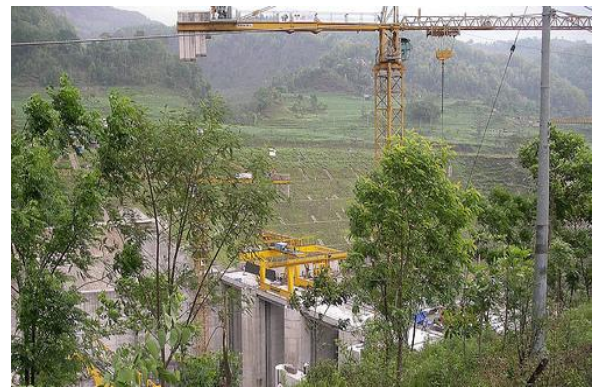
Figure 2: Hydroelectric potential being developed in Nepal
